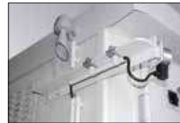
Signal siren for venting system and door opening system
